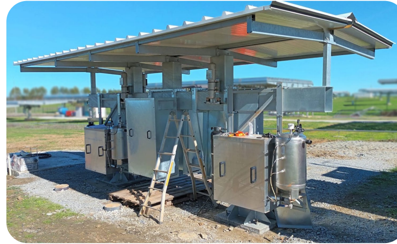
HEVO-Chain demonstrator installed in Évora
