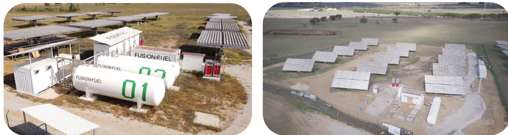
Evora Green Hydrogen Plant First Green Hydrogen Plant Live in Portugal
